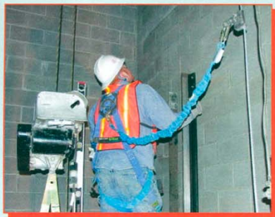
WORKER HOOKED UP PROPERLY TO LIFELINE
